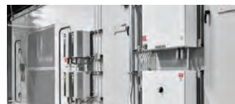
Electrical and Instrumentation
