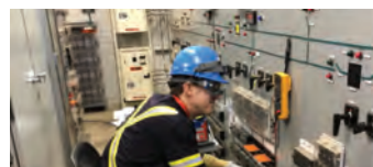
High Voltage Testing & Commissioning
